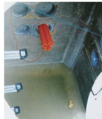
▲ Chamber of manhole with COD connected.
